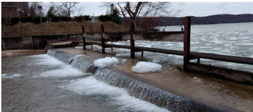
Outlet dam, March 2017: three center boards raised, west board removed, east board in place, to maximize outflow since the lake was well above winter target level. (photo: E. Hoogterp)
