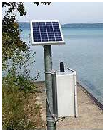
Automatic sensor monitoring lake levels at the Outlet
