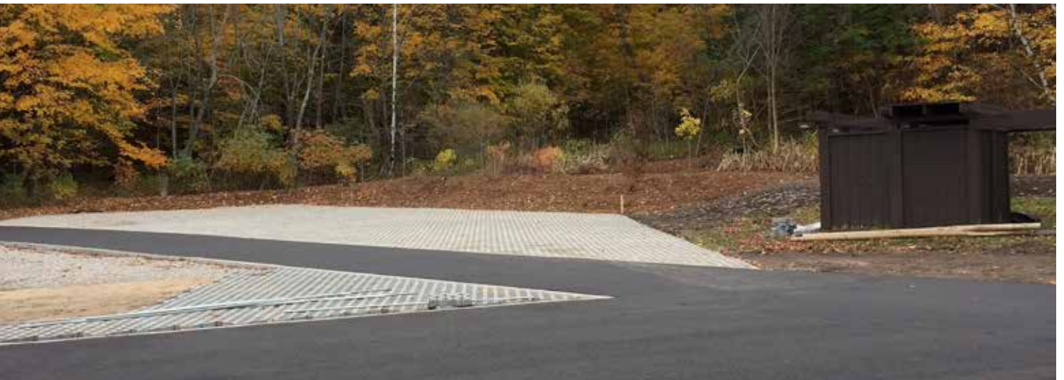
New parking area with permeable pavers, rain garden in the wetland in background, old restrooms in temporary location to right, November 2016 (photo: J. Buzzell)
