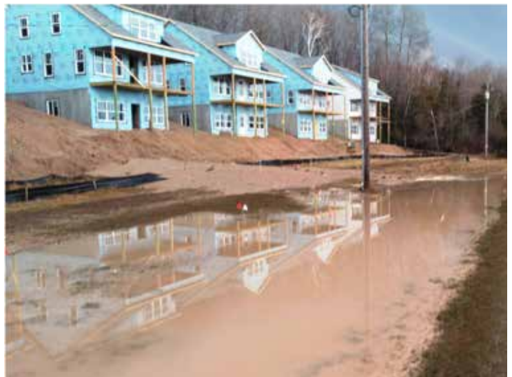
Overflow breach in protective silt fence and erosion following storm, April 5, 2023; Betsie Valley Trail at right (photo EGLE)
